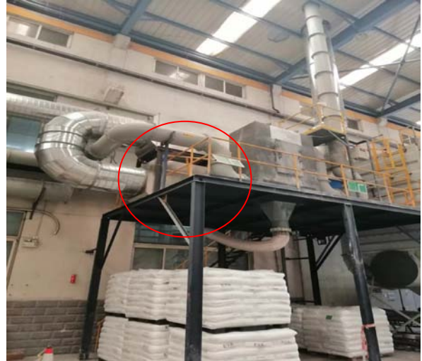
DA009#排气筒二级活性炭吸附箱
